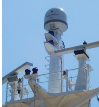
Unicom's TracVision M9 systems were installed by the vessels' electrical engineers, with activation completed in less than two hours for each antenna.
